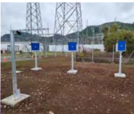
Commercial deployment for Transelec in Chile
